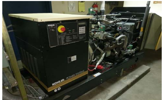
Emergency generator at Kenai Central Auditorium
